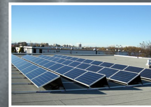
Solar-Power unit for common area
